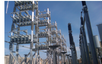
HV Shunt Bank
