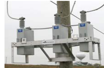
Pole-mounted Capacitor Bank
