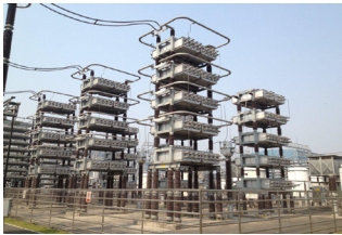
Series Capacitor Bank
